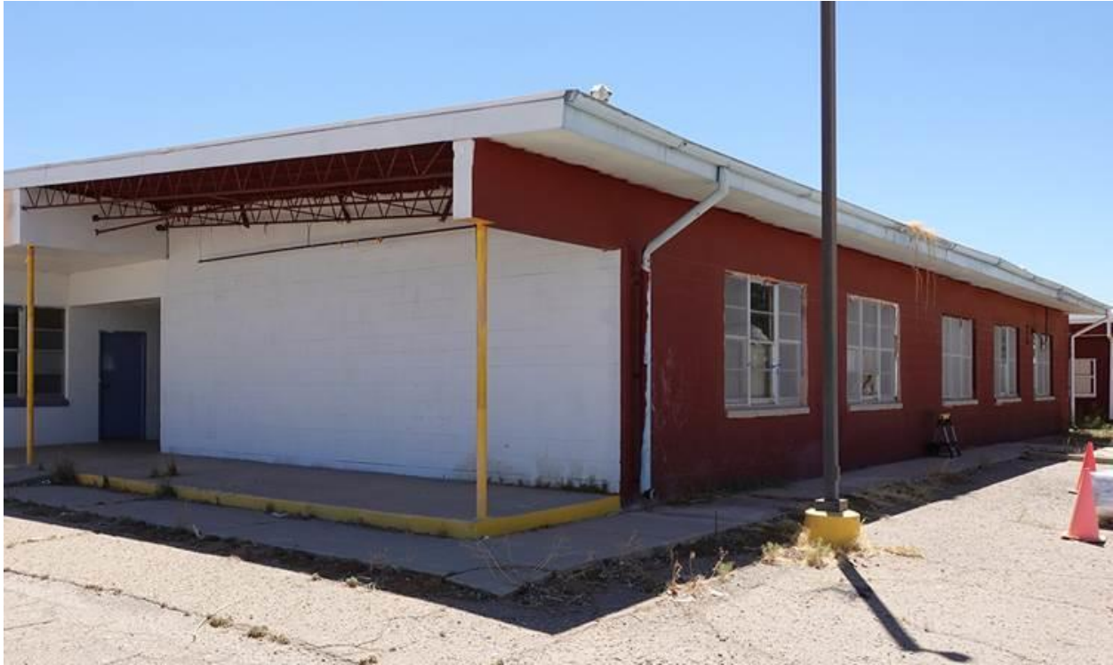
Santa Rosa Ranch School Main Classroom Building (to be demolished and replaced)
