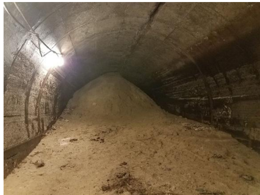
Figure 3: Fort Laramie Canal Tunnel Collapse | Source: Brierley Associates
