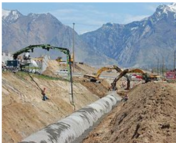
Picture 1: Piping of the Provo Reservoir Canal in Utah, Source: Bureau of Reclamation, Upper Colorado Region
