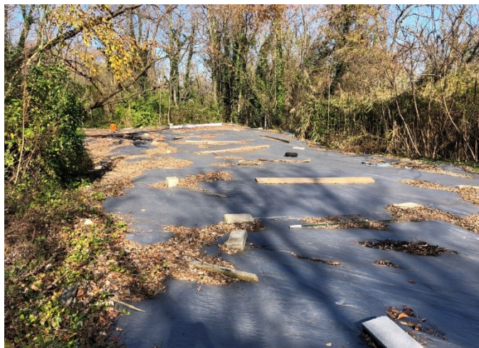
Hot spot covered with heavy duty tarps during the Sauer Dump site inspection in November 2020.
