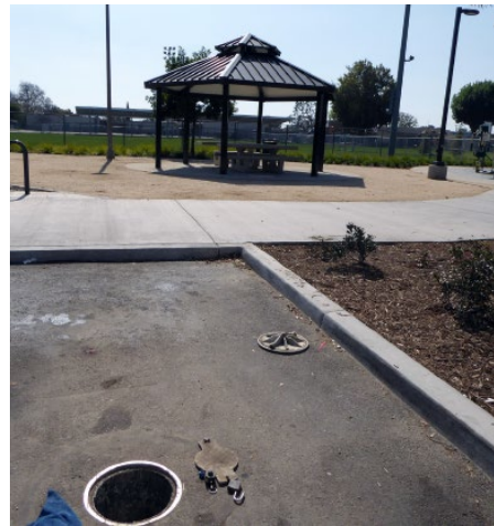
Groundwater Monitoring Well
