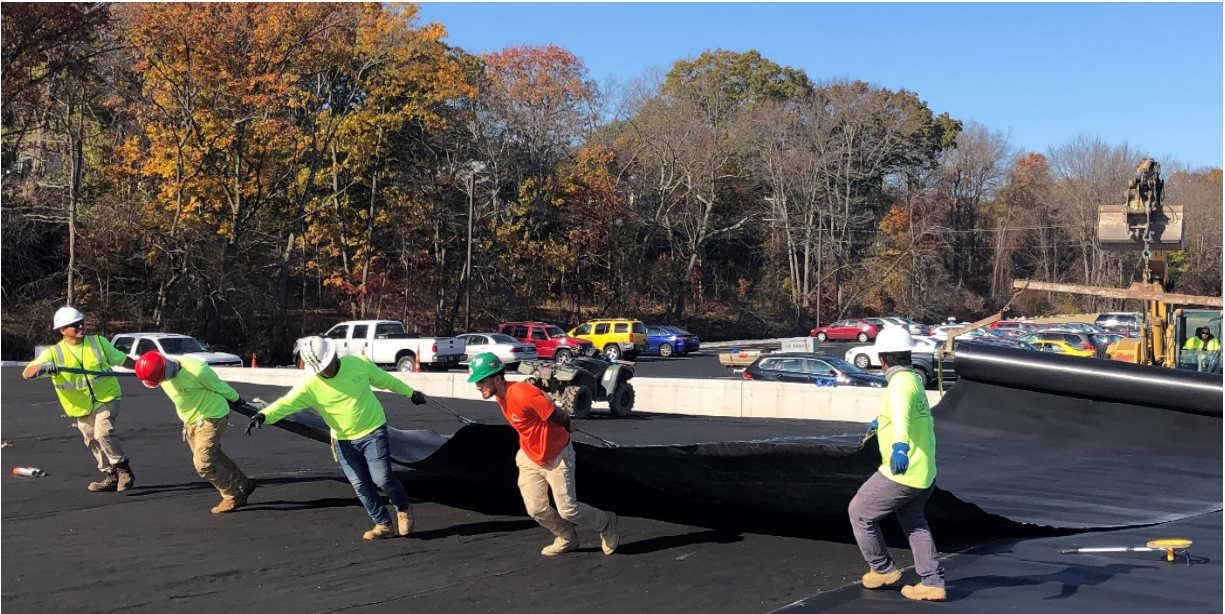
Installing the cap liner on the source area at the Centredale Manor site.
