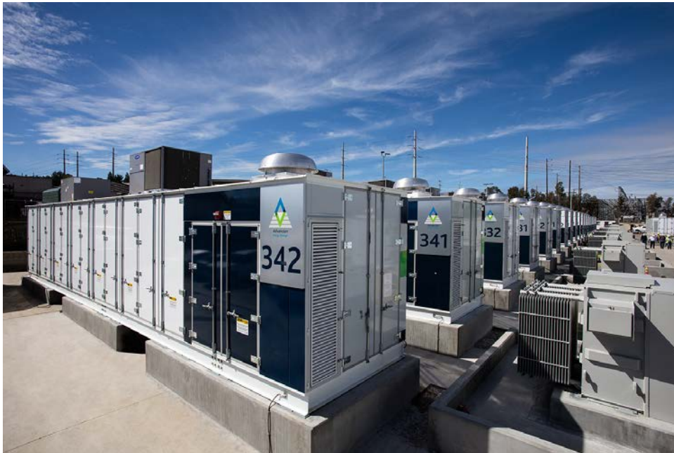
30 MW SDG&E Advancion Energy Storage Facility – Escondido, CA
