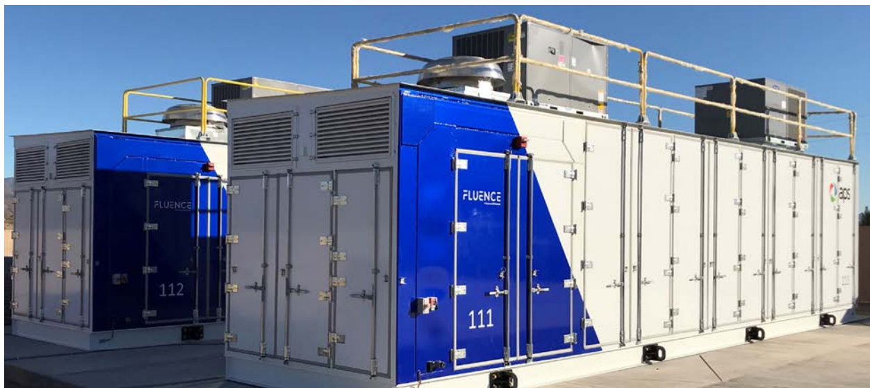
2 MW APS Advancion Energy Storage Facility – Punkin Center, AZ
