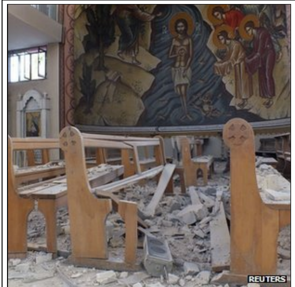
A church in Homs, damaged during fighting between security forces and rebels. (Photo: Reuters)
