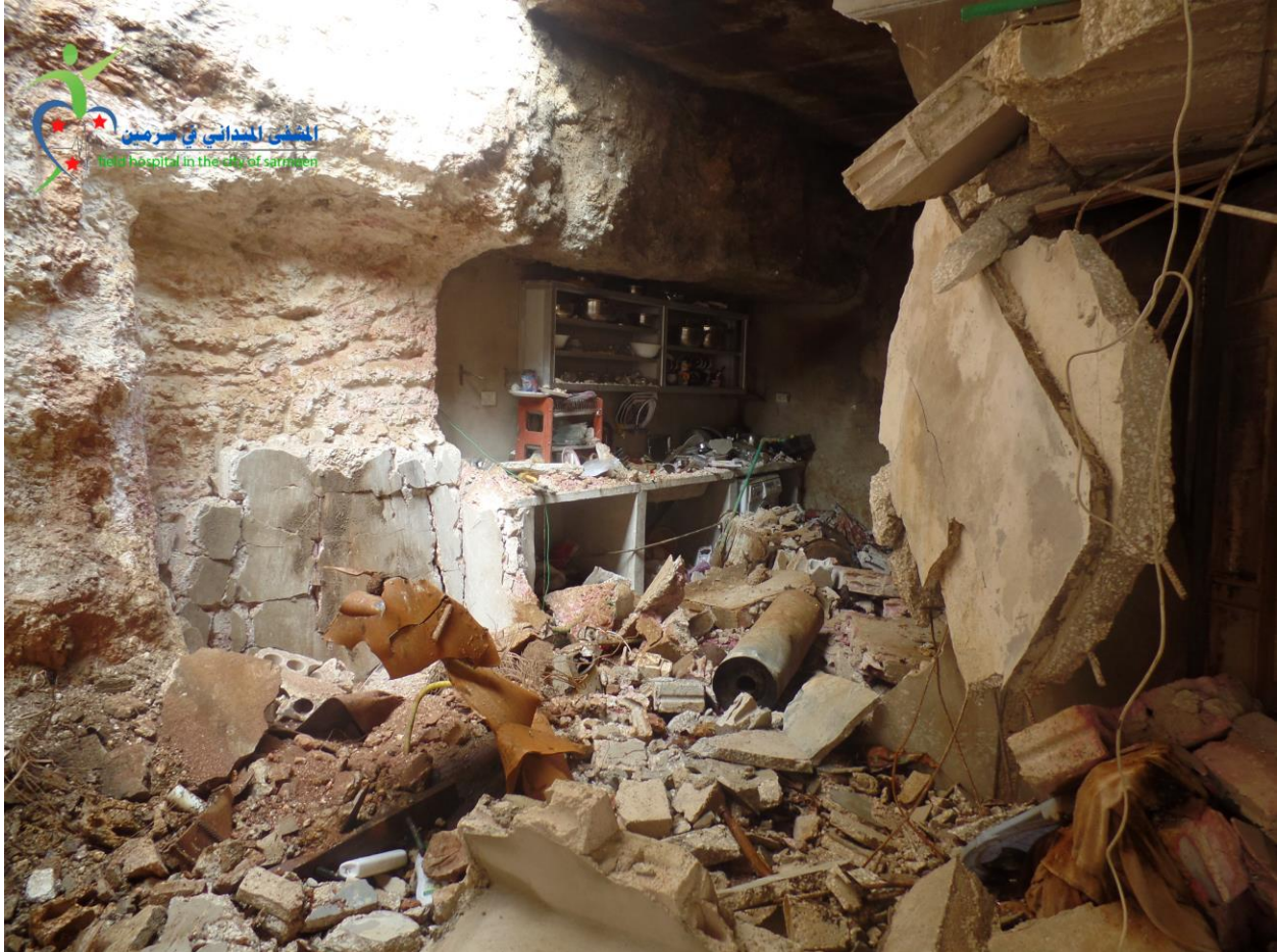
The basement of the Taleb family's house after being hit by chlorine-filled barrel bomb, taken the day after the attack
