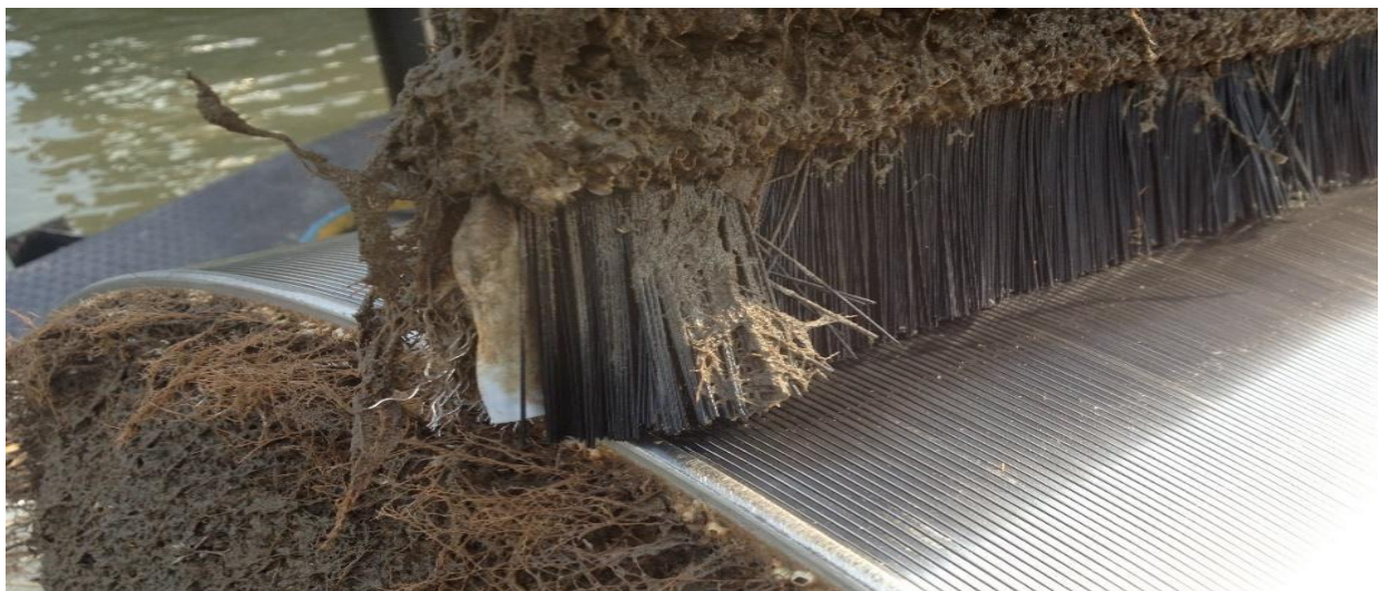
Figure 2-13: ISI mechanical brush-cleaned screen operating in Hudson River (Intake Screens, Inc. Report)
