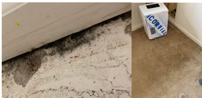
Water penetration in the same corner of New Heritage Park homes
