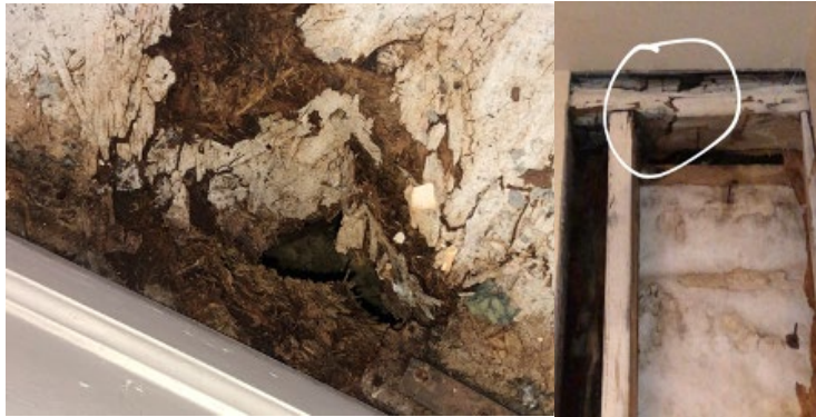
Rotting wood on the floor (L) and in the wall (R)
