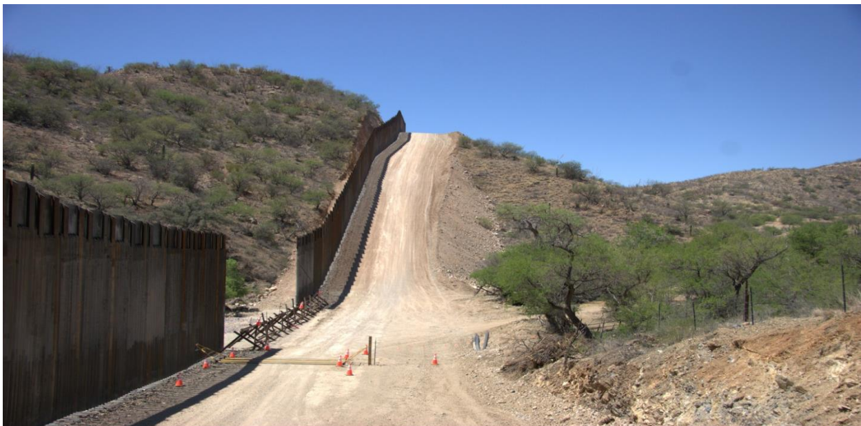
Large wash crossings like this one on our ranch at the international boundary were left unfinished when wall construction was halted and are currently an open door for Cartel border crossers.
