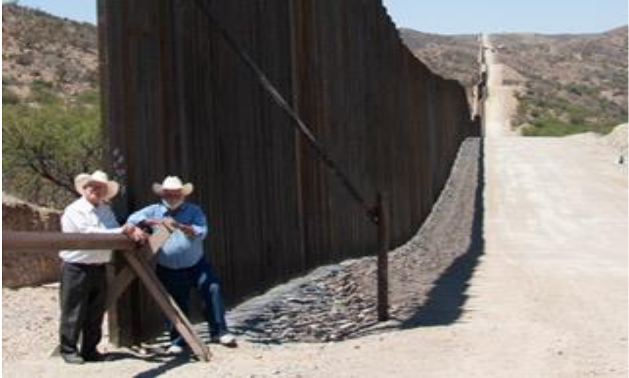
Jim Chilton and cousin Jerry Chilton at the end of Trump wall on our ranch. Large gaps were unfinished and fiber optic cable, electronics, sensors and cameras were not installed when the wall construction “stop order” was given.
