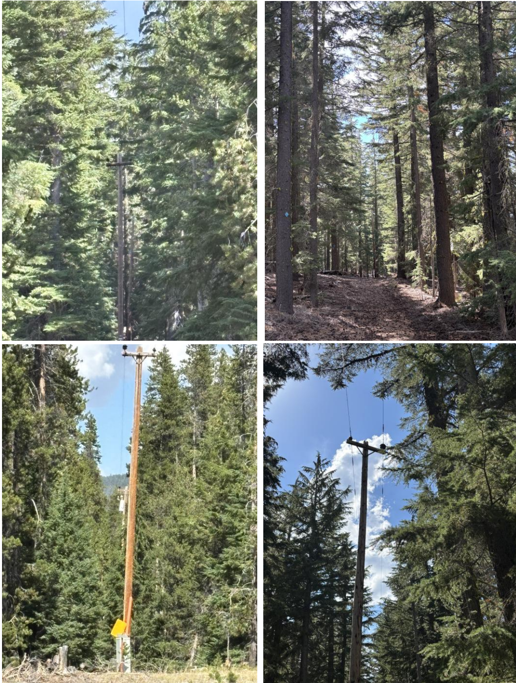
Trees encroaching on electric distribution infrastructure, Newberry National Monument
