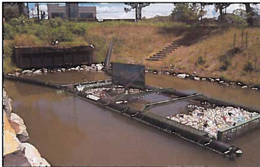
Photo of a Bandalong™ litter trap designed and installed by Stormwater Systems of Cleveland, GA, along a tributary to the Anacostia River. The District has funded the installation and maintenance of nine structural controls like this one from funding sources such as the Anacostia River Clean Up and Protection Fund generated from the five cent fee on single-use plastic retail bags.
