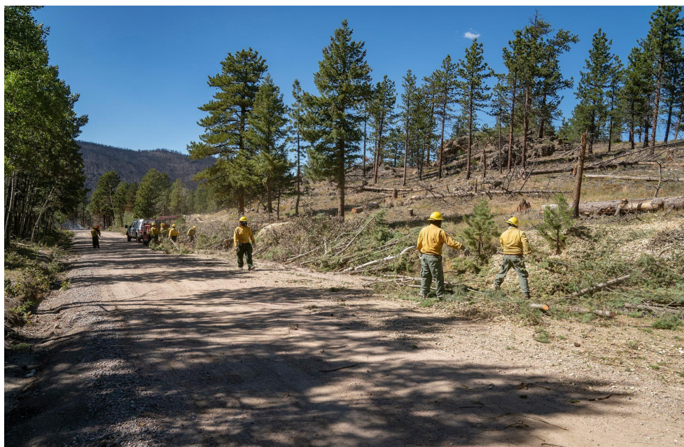
Figure 13: Roadside clearing and brushing to make the road defensible. This work along POD boundaries improves its potential for control.
