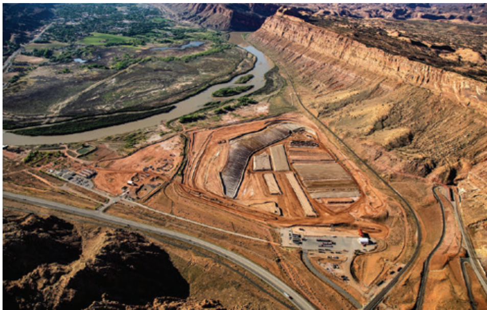
Cleanup of the Atlas Uranium Mill, on the bank of the Colorado River in Moab, Utah, is expected to cost around $1 billion by 2032. JIM HODDENBACH, MOAB URANIUM MILL TAILINGS REMEDIAL ACTION (UMTRA) PROJECT, U.S. DEPARTMENT OF ENERGY
