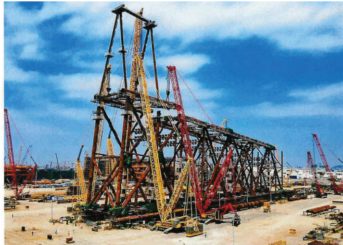
Workers assemble a jacket for an offshore oil platform at a construction site in Zhuhai, China. Source: Cnooc
