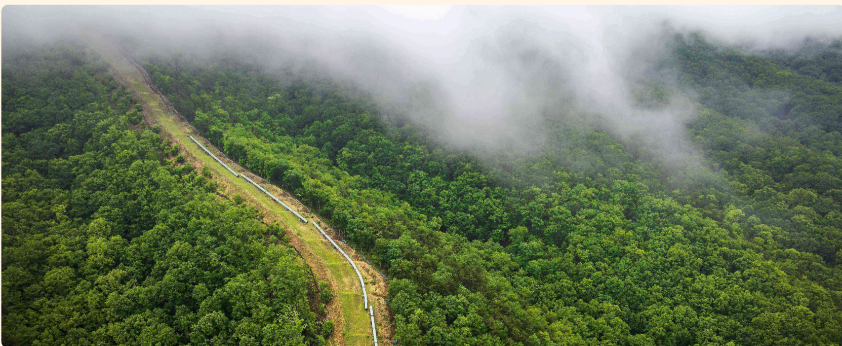
The path of the embattled Mountain Valley Pipeline runs more than 300 miles from West Virginia into Virginia with a proposed extension into North Carolina, including this portion cutting through the Jefferson National Forest in Virginia. ©Mason Cummings
