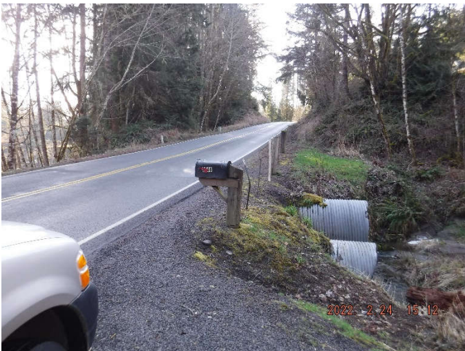
Roadway approximately a week prior to washout
