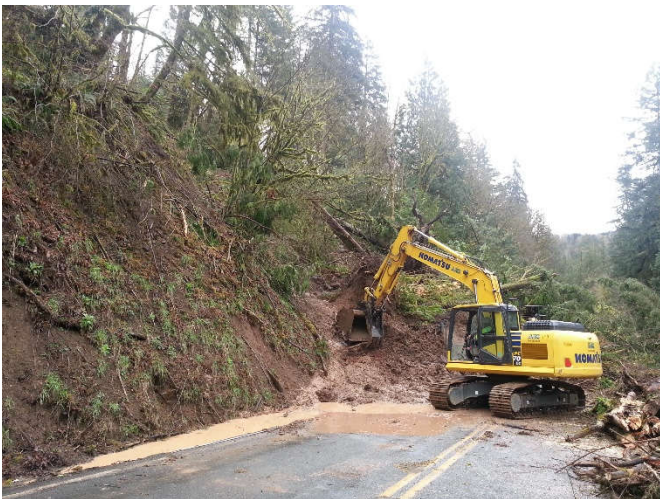
Roadway closed by slide material
