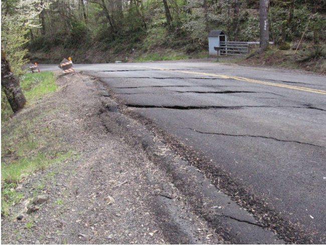
Section of roadway that needs to be frequently paved
