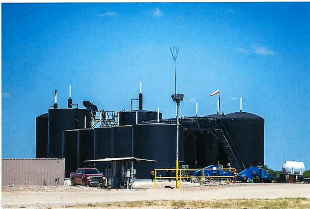
Fracking wastewater tanks near Big Wells, Texas. Sergio Flores for The New York Times
