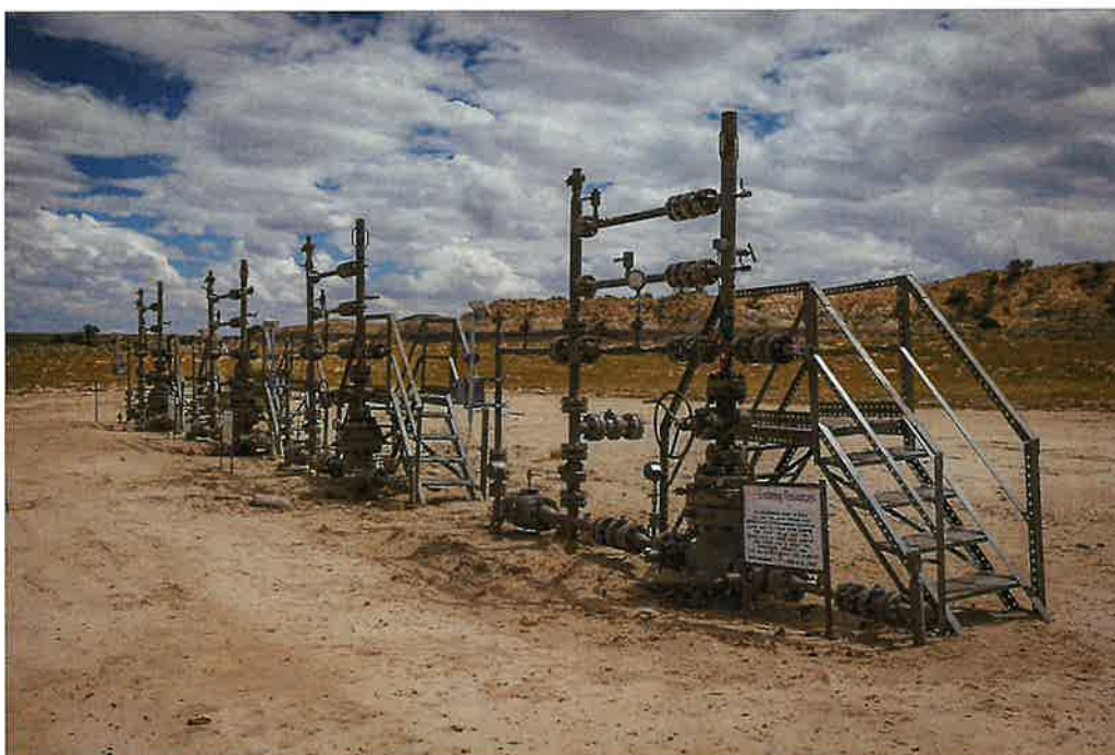
A gas well near the Atencio home. Sharon Chischilly for The New York Times
