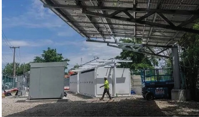
A solar battery energy storage site in the Bronx, part of a test program to support New York's transition to renewable energy sources. Credit—Hiroko Masuike/The New York Times
