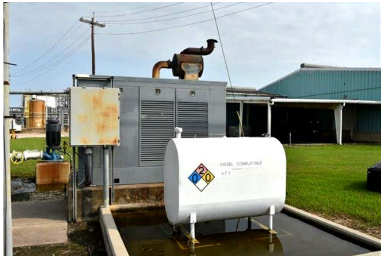
Inundated power generator at the Arkema facility following the chemical disaster. Source: U.S. Chemical Safety and Hazard Investigation Board
