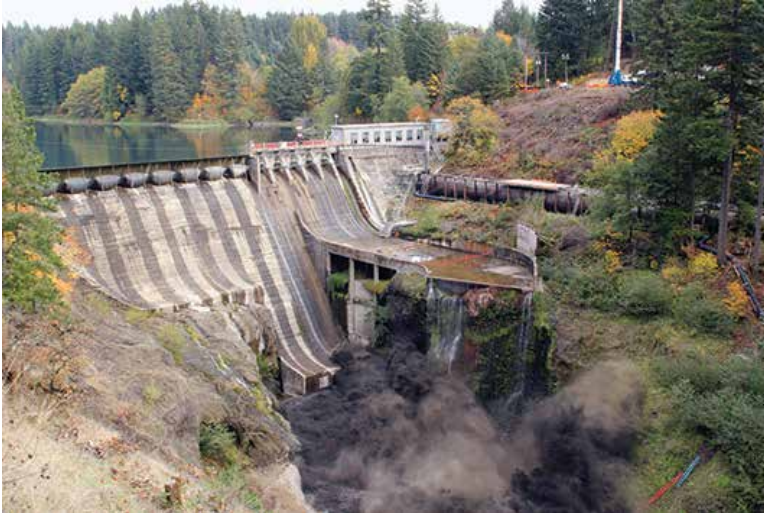
The blast at the base of Condit Dam that initiated the breaching of this 100-year-old structure on the White Salmon River.
