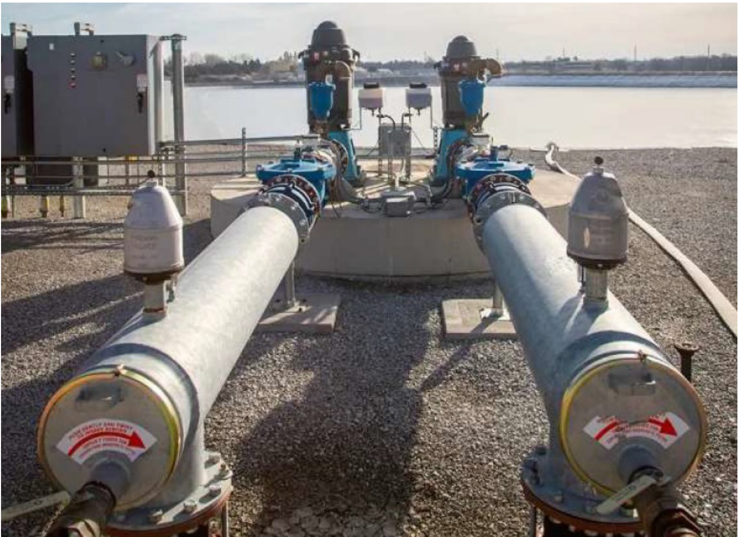
Pumps part of the aquifer storage and restoration project to remove excess nitrogen. Photo credit to City of Hastings, NE.
