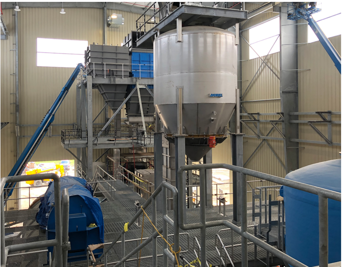
Interior of the biosolids reuse processing facility at the Village Creek Water Reclamation Plant in Fort Worth, TX. Photo Credit: Texas Water Development Board.
