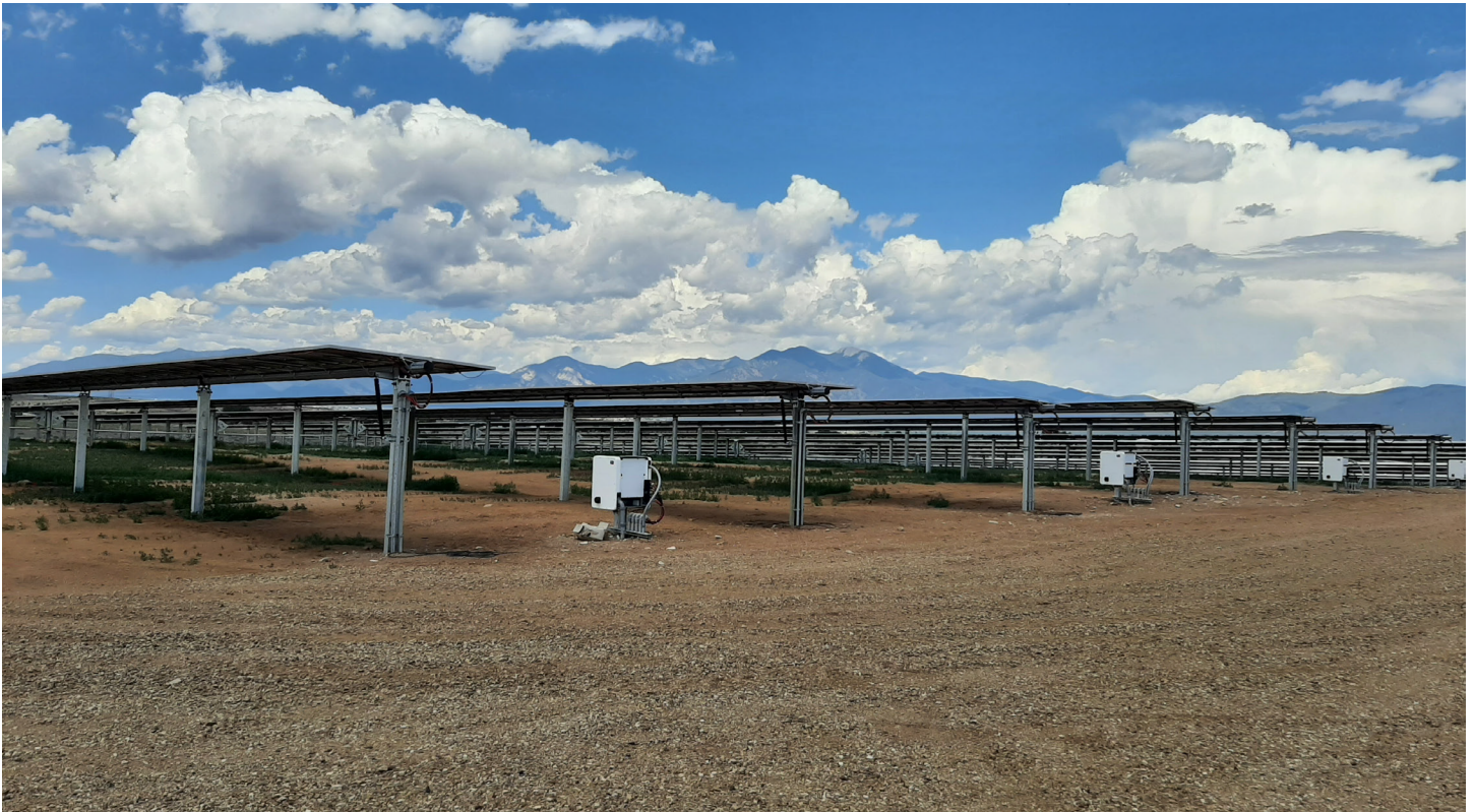
Solar array providing power at the Town of Taos wastewater treatment plant. Photo credit to New Mexico Environment Department.
