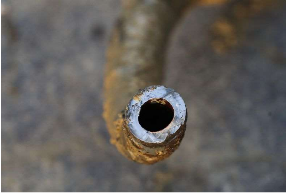
An old lead service line is removed from a home in Galesburg. Pipes known as service lines connect homes to municipal water supplies. Galesburg is planning to replace all of its lead service lines by the end of the year. (Jose M. Osorio / Chicago Tribune)
