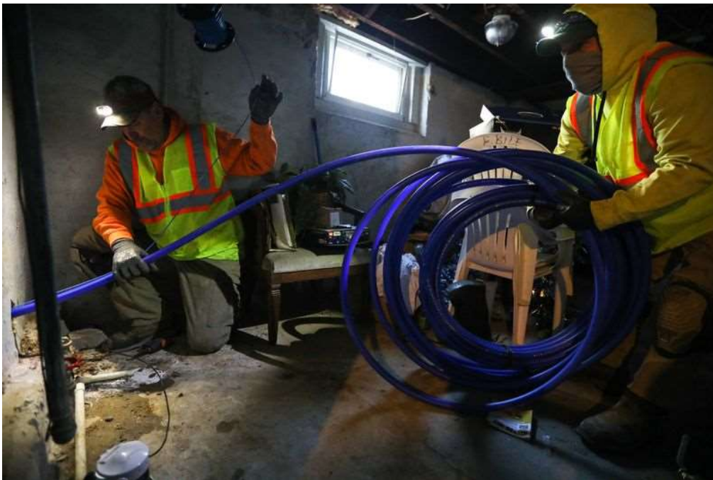
Tom Gorham, left, feeds new polyethylene tubing through the opening where the lead service line was in a home in Galesburg. (Jose M. Osorio / Chicago Tribune)
