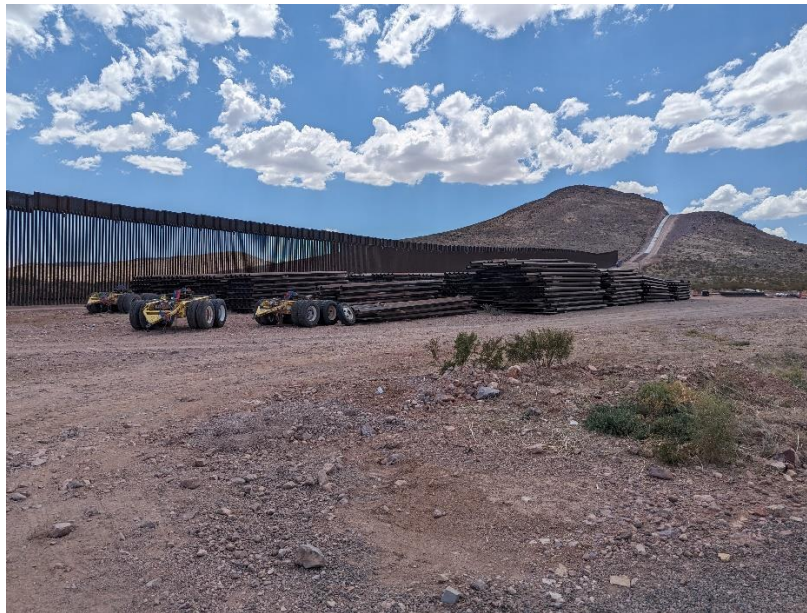
Wall panels left behind near \frac{3}{4} mile gap
