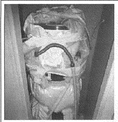
Tank wrap is unprofessionally installed.
