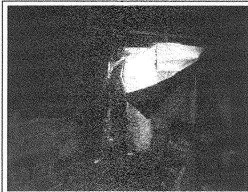
A broken basement window which someone tried to cover with plastic. Note the large holes by the lower left corner of the window where bricks were crumbling. This window represents a large area of air infiltration which should have been addressed as part of weatherization.
