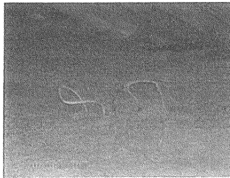
Unit # 6, Job Identifier ARRA-A-901, exposed spliced wires in attic.
