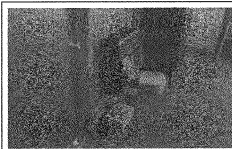
Unvented gas space heater left in bedroom, gas hooked up, pilot burning. Note rags substitute for door sweep in bottom left of photo.
