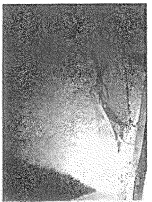
Unit #2, Job Identifier ARRA-C-199, exposed spliced wires
