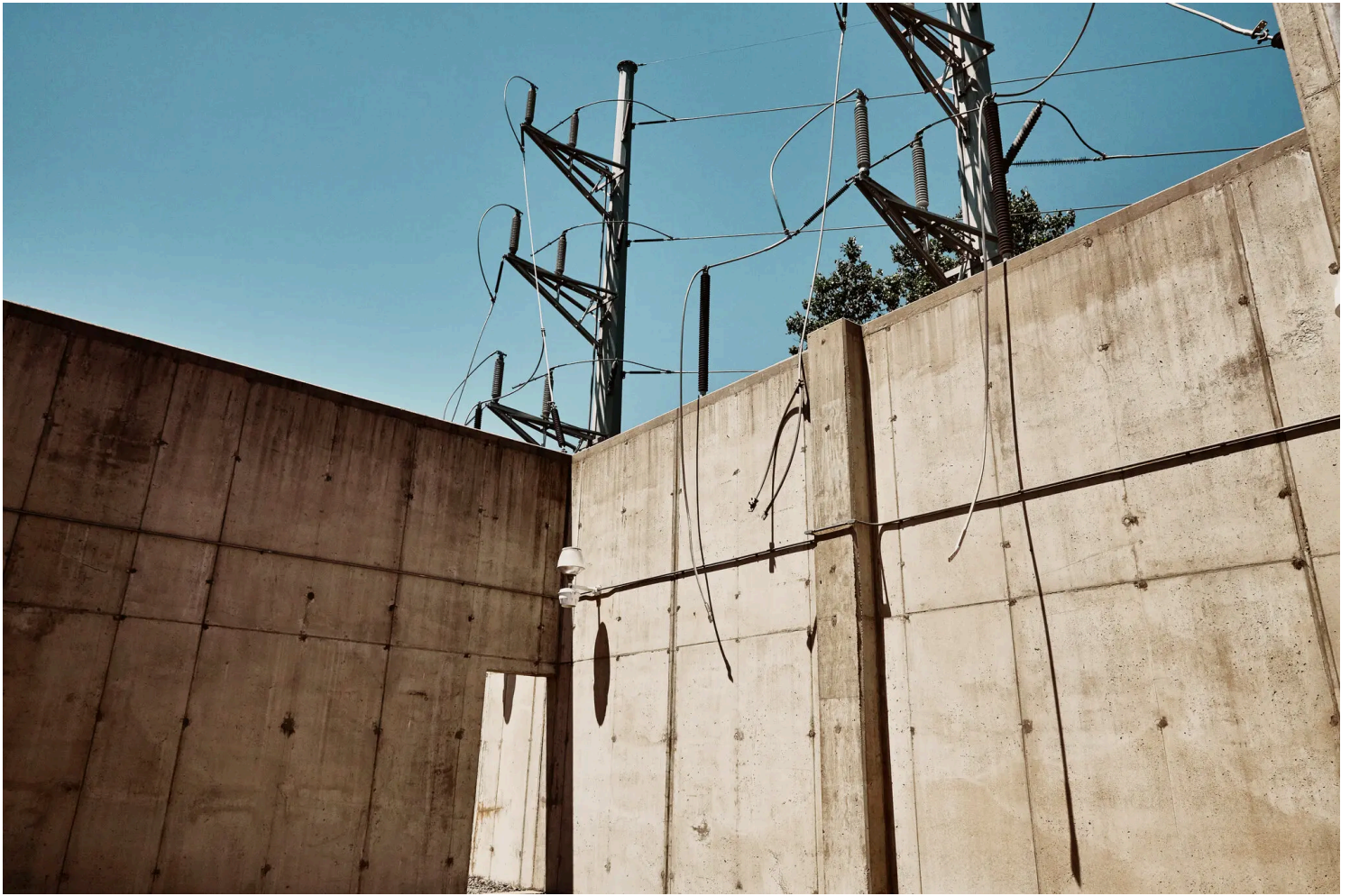
A building that formerly housed transformers at the Brayton Point Power Station, a decommissioned coal plant that is being repurposed to link a wind farm to the Massachusetts power grid. Simon Simard for The New York Times
