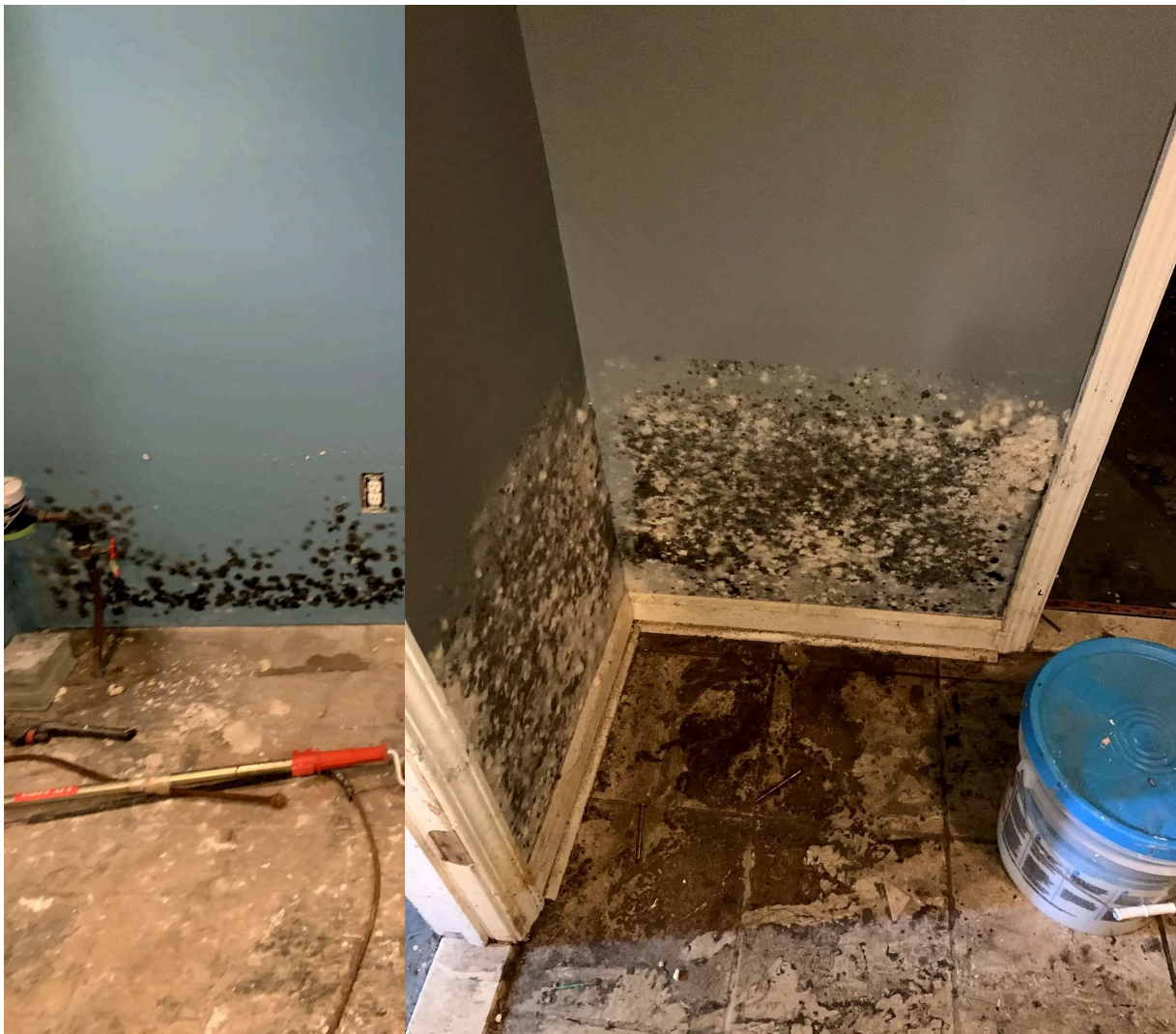
Severe basement flooding in 2021 left toxic black mold in Wilma Price's home in the Jefferson Chalmers neighborhood. To remediate the mold, parts of the walls were ripped out.
