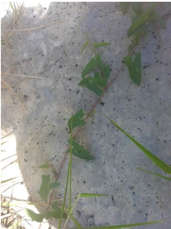
Figure 32: Coal Pieces Located on Large Rock Directly Under Railroad Bridge Crossing Clinch River
