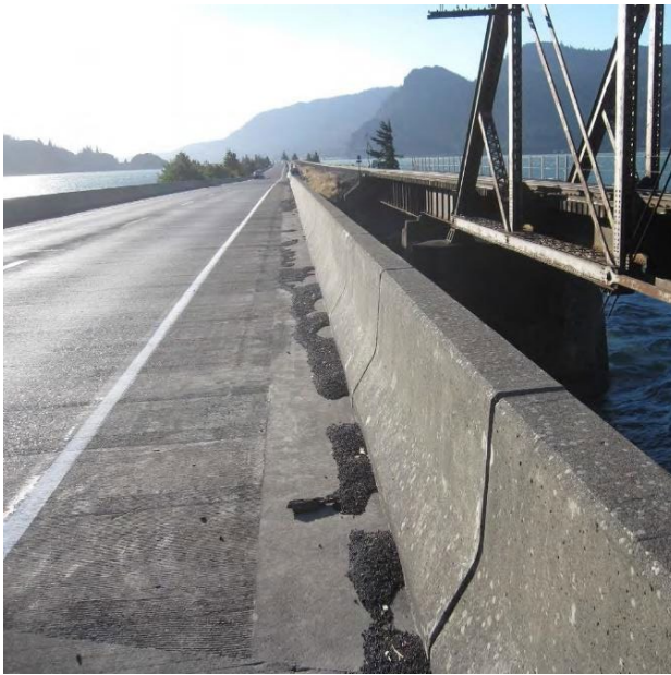
Figure 5: Coal Accumulations on Roadway Bridge over Drano Lake, Adjacent to BNSF Bridge over Same Waterway
